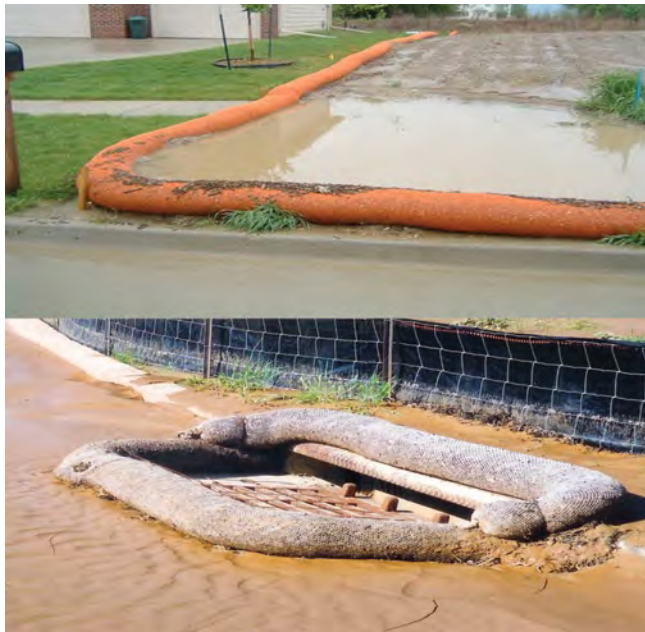
Figure 9.14. Compost in filter socks reduces runoff and protects stormwater quality. Photos courtesy of Rod Tyler, Filtrex International LLC.
