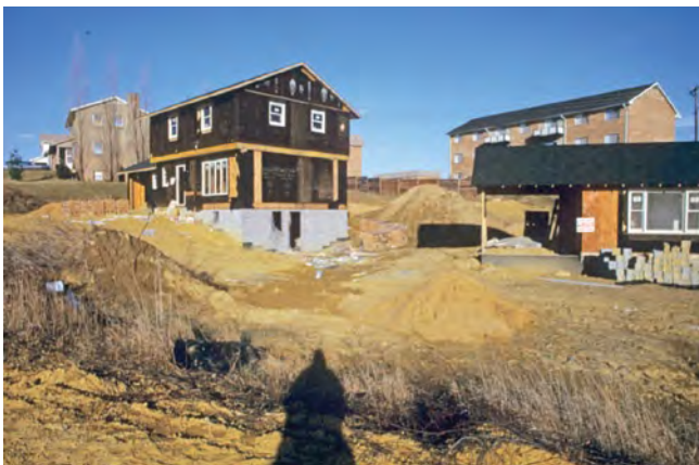
Figure 3.2. Typical soil disturbance in subdivision during construction. Each lot is graded out (cut and filled) to approximately level the area immediately surrounding the house. Note large amounts of sand and other construction debris that will more than likely be graded out and incorporated into fills.
